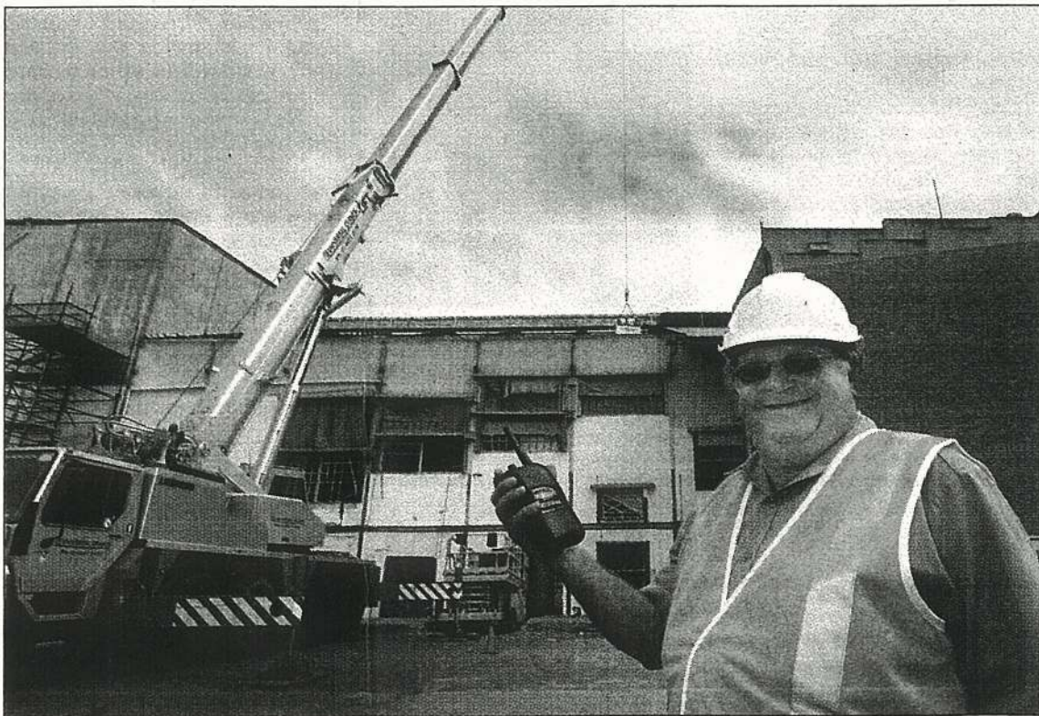
HAPPY MEMORIES: Ray Busby supervises demolition work at the Wintergarden Theatre yesterday afternoon. Picture by CHRIS ISON.
