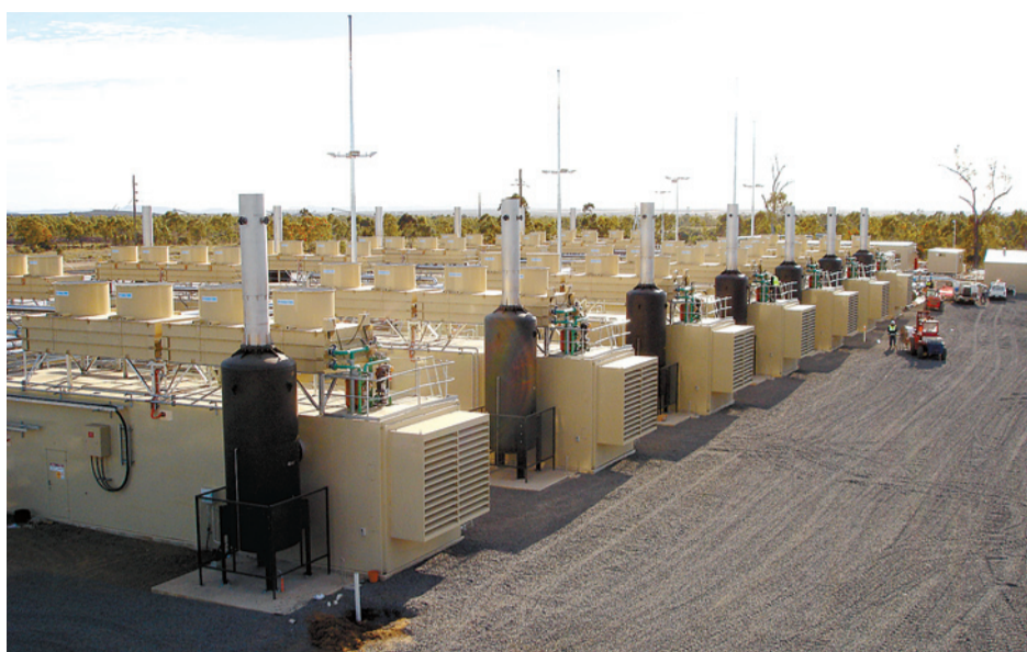
Above: Jenbacher engines located on the 15 x 64m 2 engine bases
